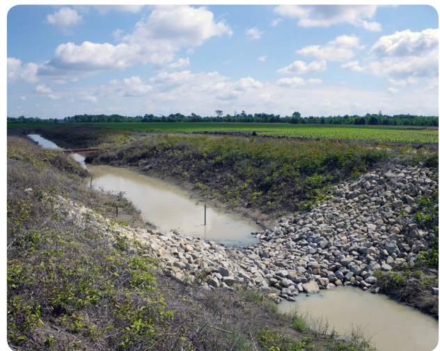
Water Control Structures Improve Water Quality
